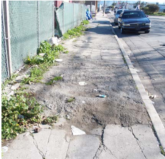
Sidewalk repair is necessary throughout Chinatown.
