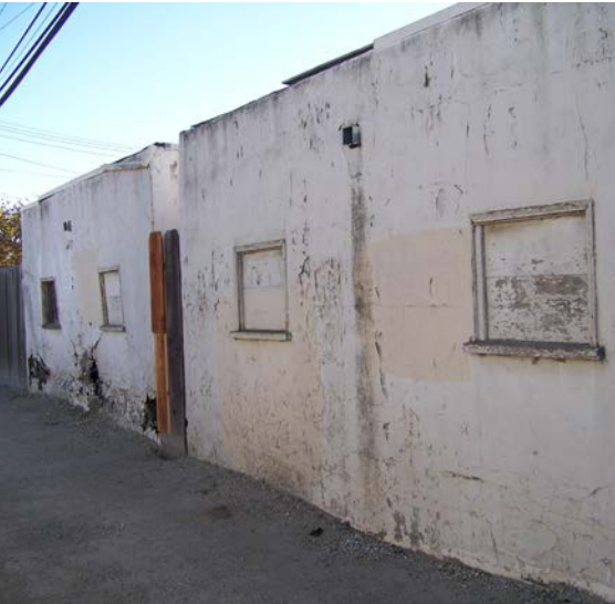
Desinvestment and deterioration is visible in Chinatown's built environment.
