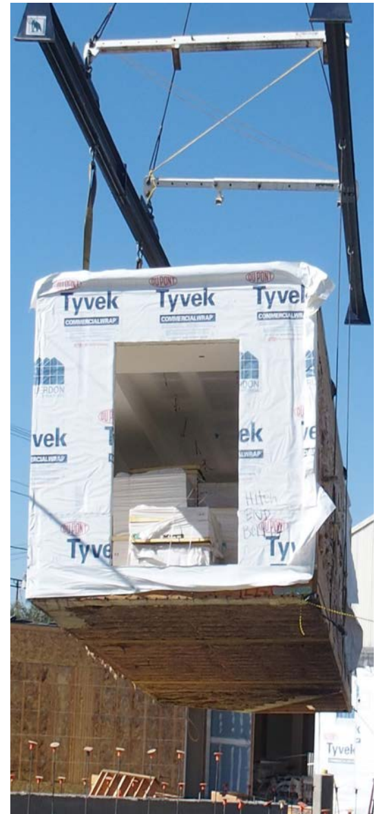
Hikari Apartments modular unit being dropped into place along the building’s foundation.
