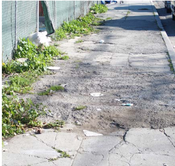
A sidewalk in Chinatown in need of serious repairs.
