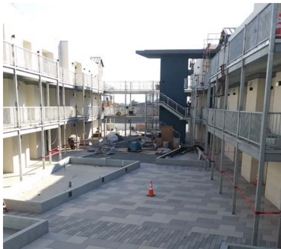
Courtyard and community open space at future Moon Gate Plaza project, currently under construction.
