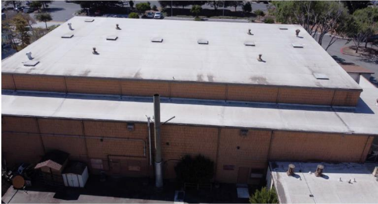
4. North facade; windows to be replaced, old boiler flue to be removed, service yard repaved and graded scope items SR6, SR12
