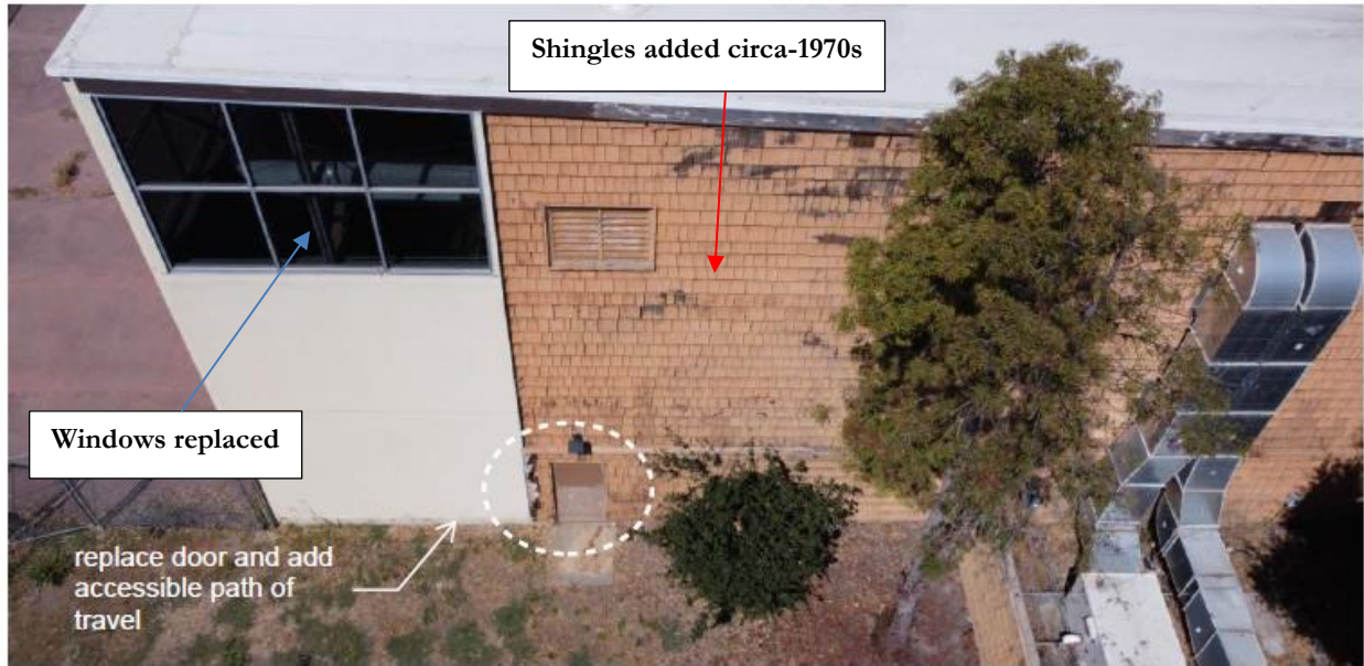
1. East Facade showing deteriorated wood shingles, Scope item SR2, SR9
