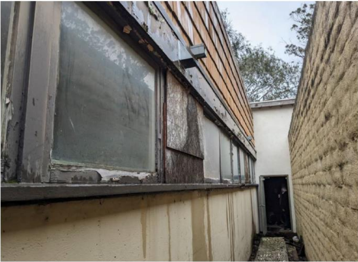
10. Deteriorated windows, exposed roof scuppers with no rainwater leaders, existing CMU screen wall to be removed; scope items SR5, SR6, SR19
