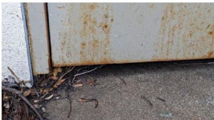
8. foundation/slab settlement at SW corner of building: scope item SR7
