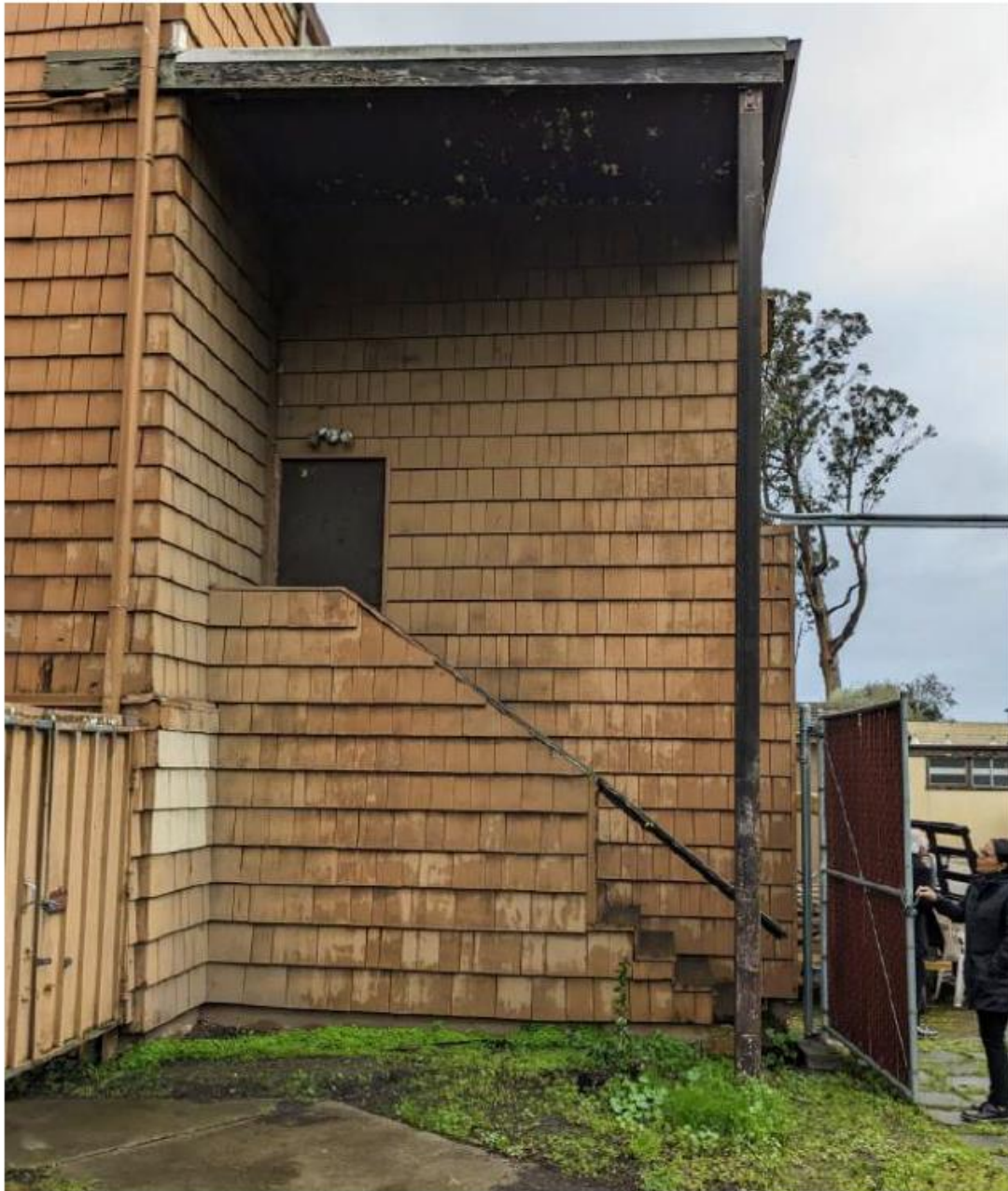
Figure 15: NE corner of building showing abandoned stair, column, door, and roof to be removed
