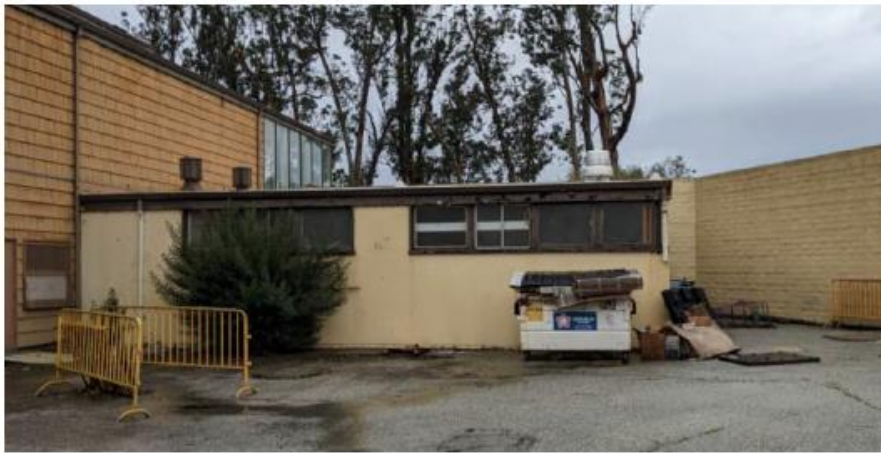
12. North service yard showing windows to be replaced and non-compliant entry doors. scope items SR6, SR12.
