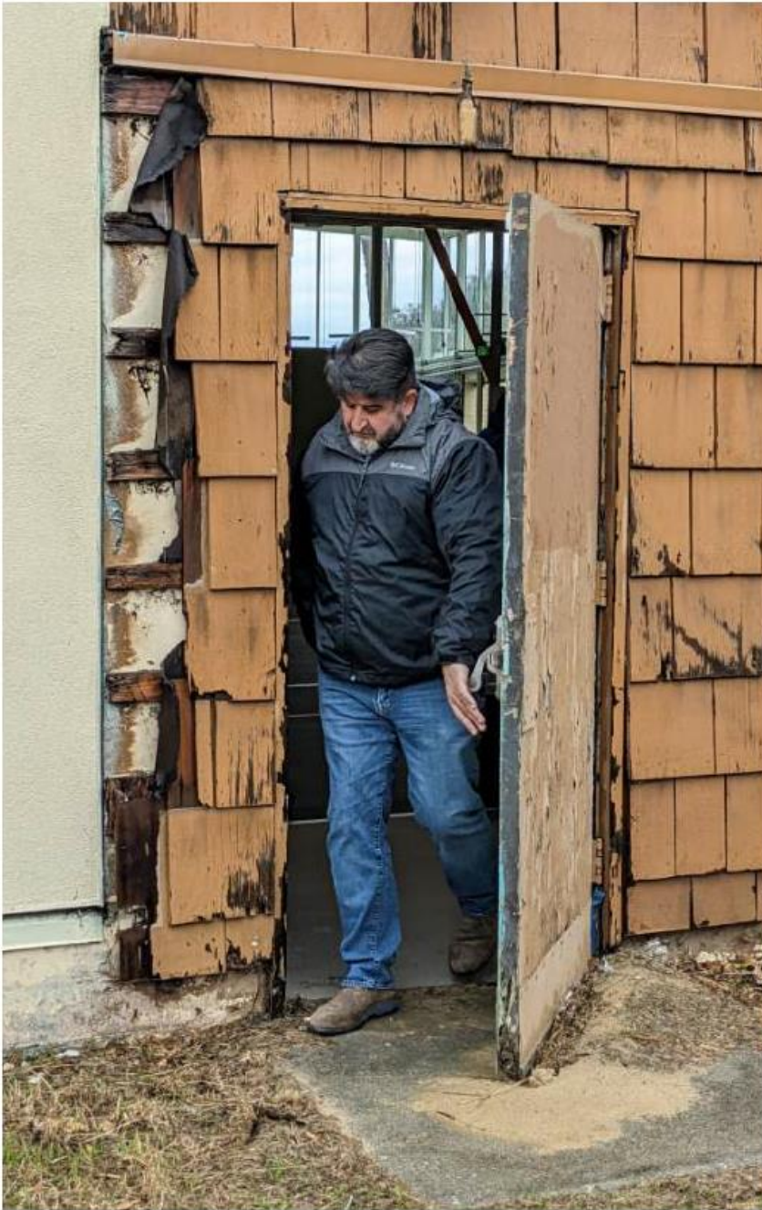
11. Deteriorated shingles and egress door at east side of building; scope item SR9.
