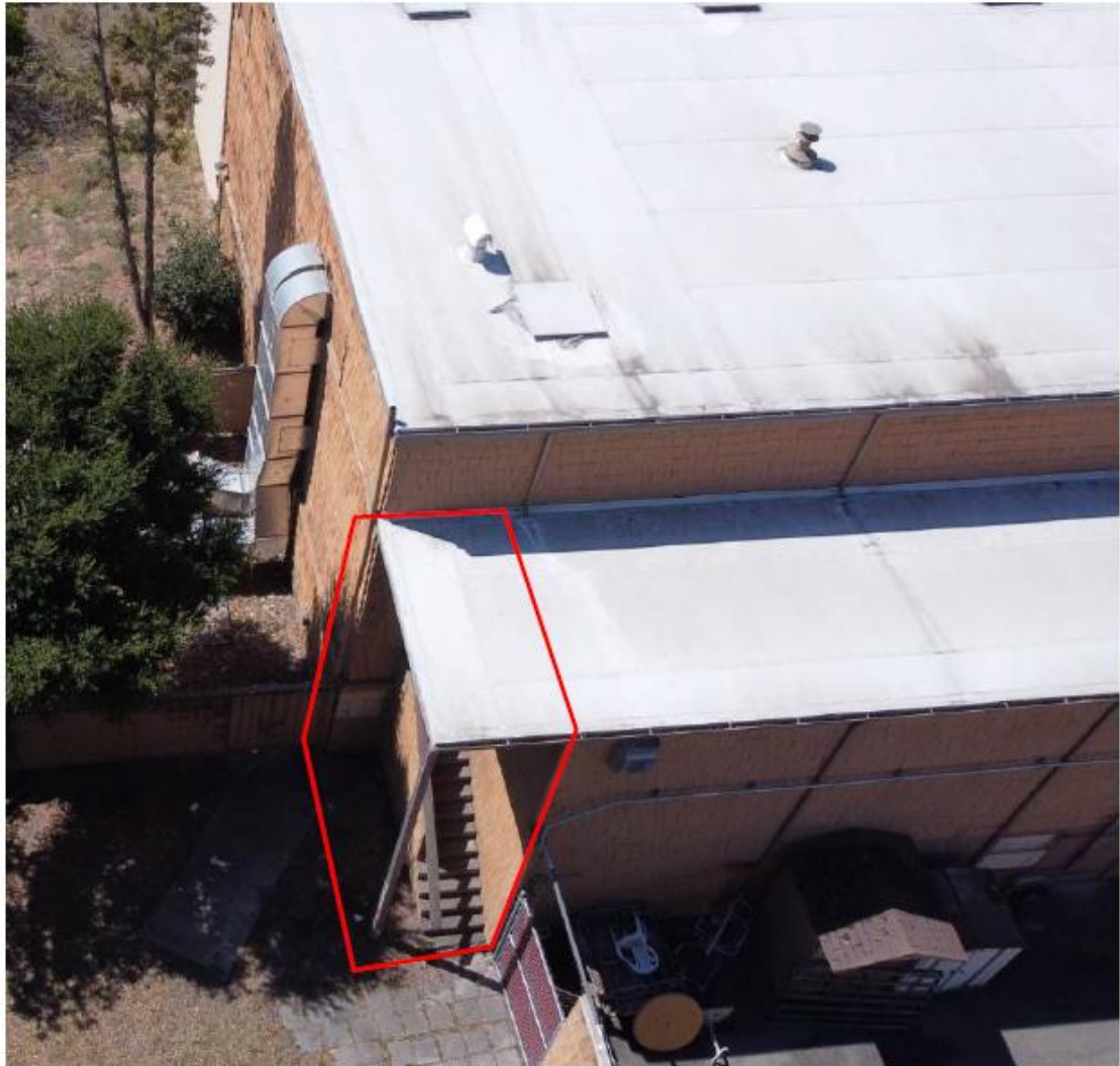
3. NE corner of building showing stair and roof structure to be removed
