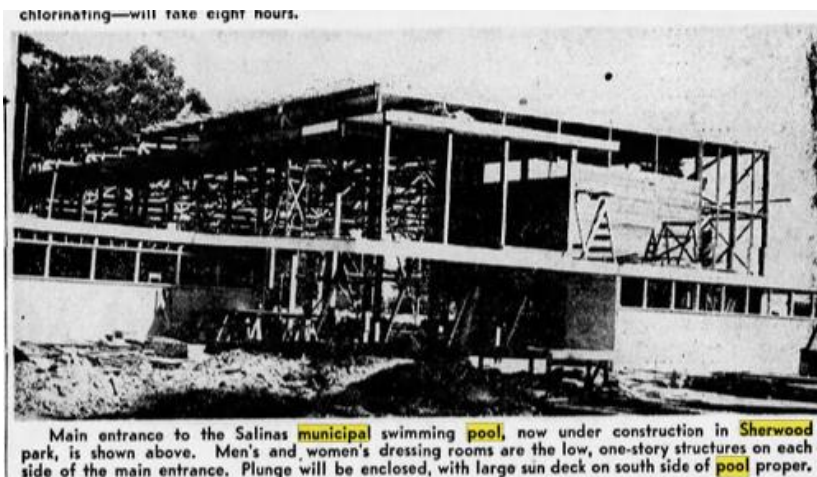
Figure 2: The swimming pool and plunge under construction ( The Californian , February 8, 1949 and April 29, 1949).
